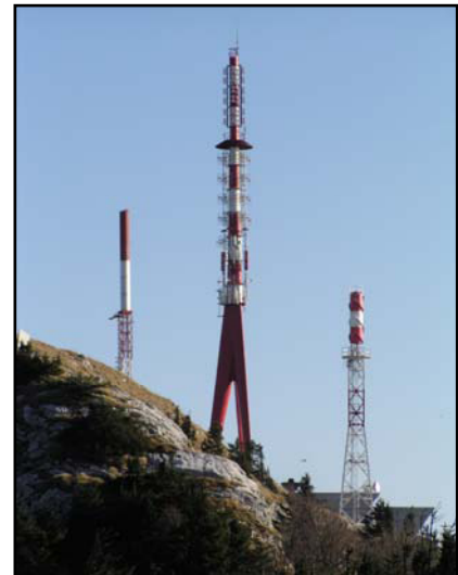
Microwave radio towers in Croatia
