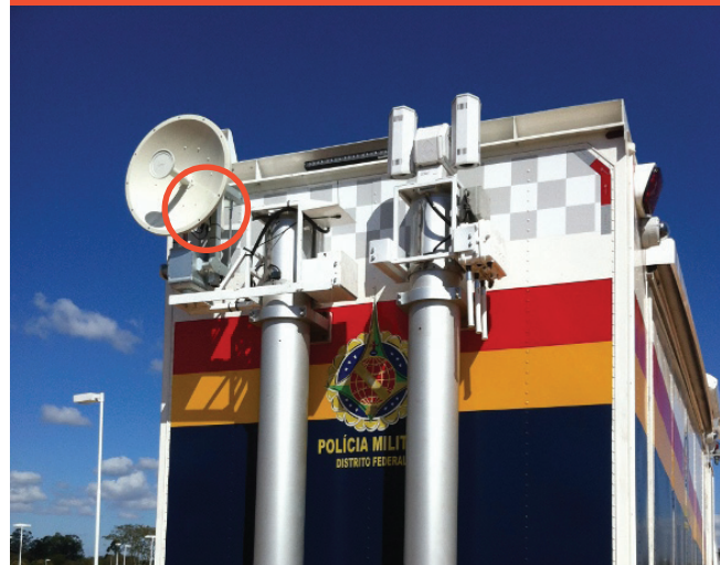
RADWIN 5000 PtMP installed on Mobile Command Center vehicle
